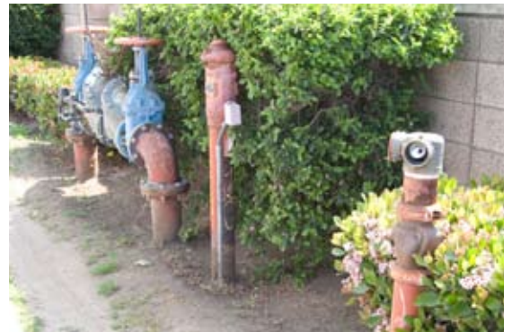
Hydrant on Pico Blvd.
