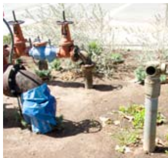
Fire hydrant at the corner of 10th St. and Santa Monica Blvd.
