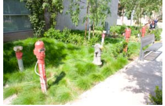
Hydrant outside the HSS.
