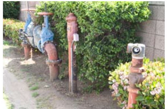
Hydrant on Pico Blvd.
