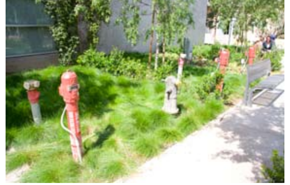
Hydrant outside the HSS.
