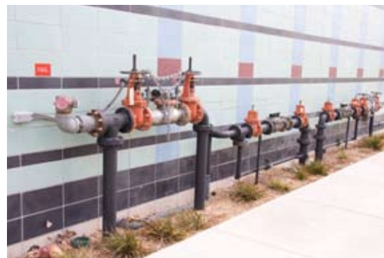
Hydrant outside the Pool.
