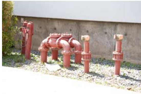
Hydrant outside the Library.
