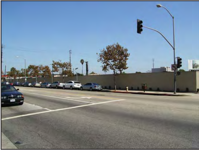
View 1: Looking southeast across Pico Boulevard toward the construction wall along the Main Campus frontage.
