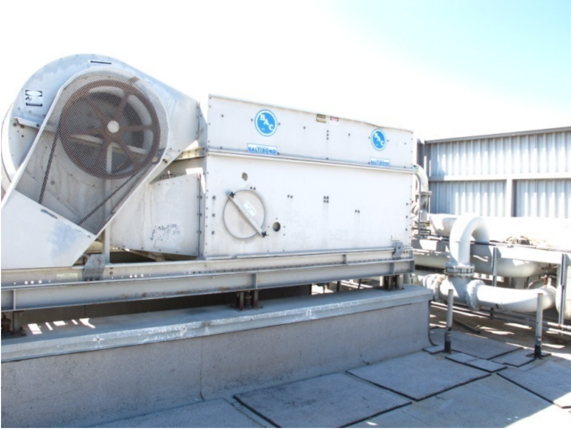
Cooling Tower for the Science Building chillers
